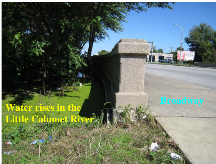
Figure 5. Water level in the Little Calumet River rose to the level of Broadway. Photo by E.P.Argyilan
